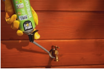
Water Faucet Penetration
