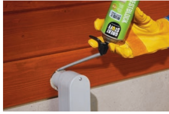
Electrical Cable Lines
