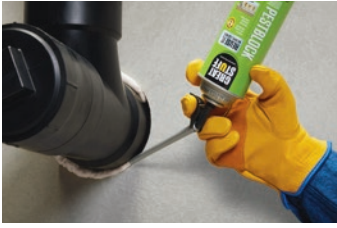
PVC Pipe Penetration
