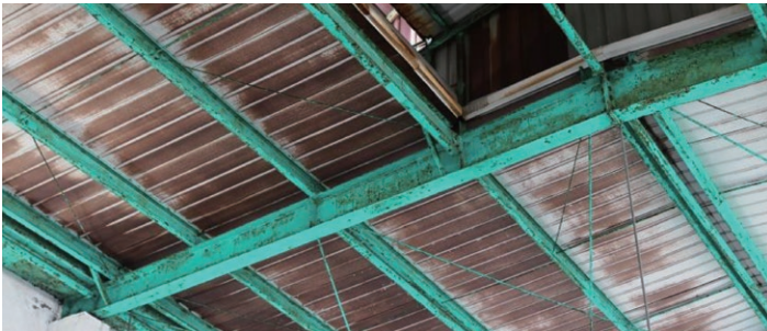
Tedlar® film laminated steel sheet roofing at far right
